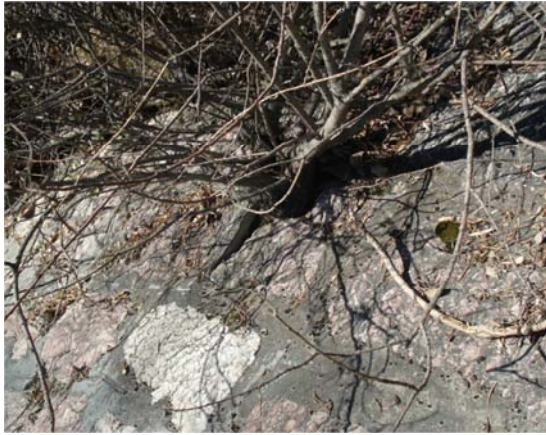
Figure 1. On going destruction of a retaining stone and masonry rip rap by a poplar cut several times. When trees are cut many times, their root system in growing faster and stronger, resulting on heavy degradations, like here with uprising of concrete joint.
