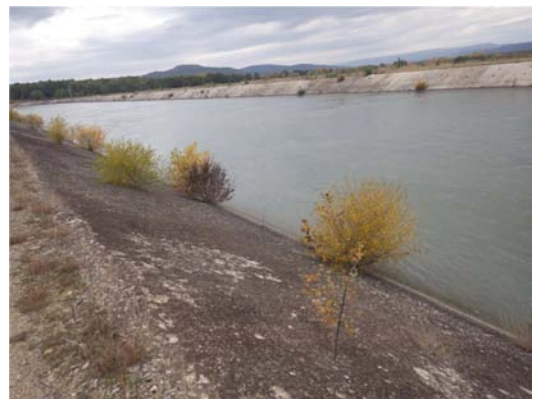
Figure 9. Colonization of concrete lock walls by young poplars which are present in drainage system breaks.
