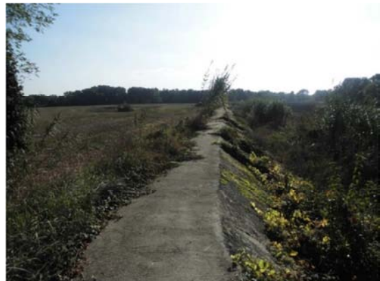
Figure 4. Entirely concreted dike where the invading species still manage to grow and deteriorate the concrete.
