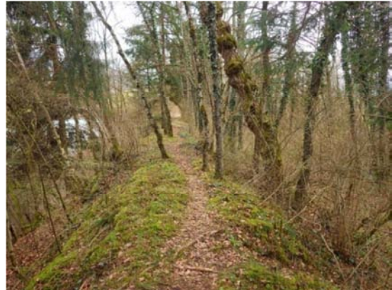
Figure 3. Entirely wooded dam presenting a critical condition in respect of the safety of the work. Trees are implanted on the both sides of the dike; most of them are dangerous in case of uprooting.
