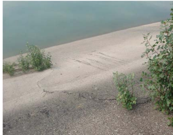
Figure 2. Apparition of numerous root suckers along a fissure on protective tar coating, generated by a shallow root resulting from the slaughtering of the main tree.
