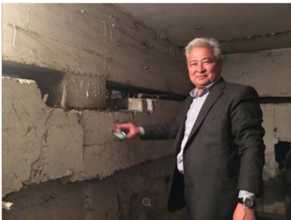
Figure 9. General view of the sliding belt in a large-panel building in Bishkek.
